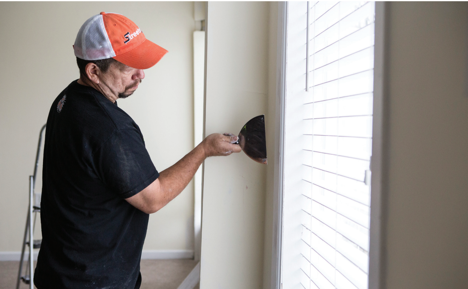
PETE MARTINEZ, OWNER OF P&A REMODELERS OF KC, works on a house in Parkville, Mo. Martinez has seen a surge in home remodeling the last few years
