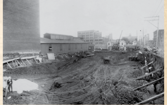
July 1922 picture of the Oklahoma City Branch construction site. Photo courtesy of Bank Archives.
